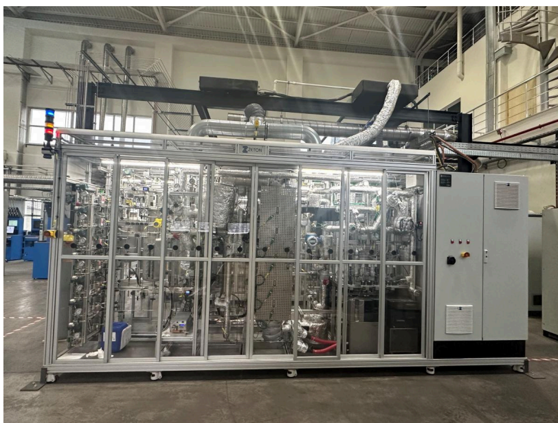
The TRL 5 pilot plant on the premises of Tüpras. Source: the project's website.
