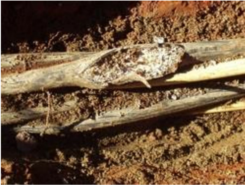
Cable line failure.
