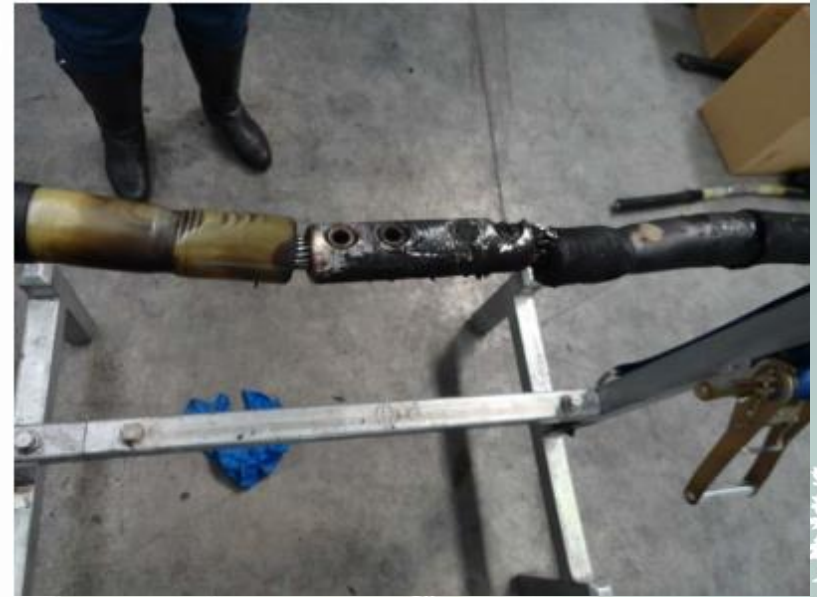
An overheated connector in a failed cable joint.
