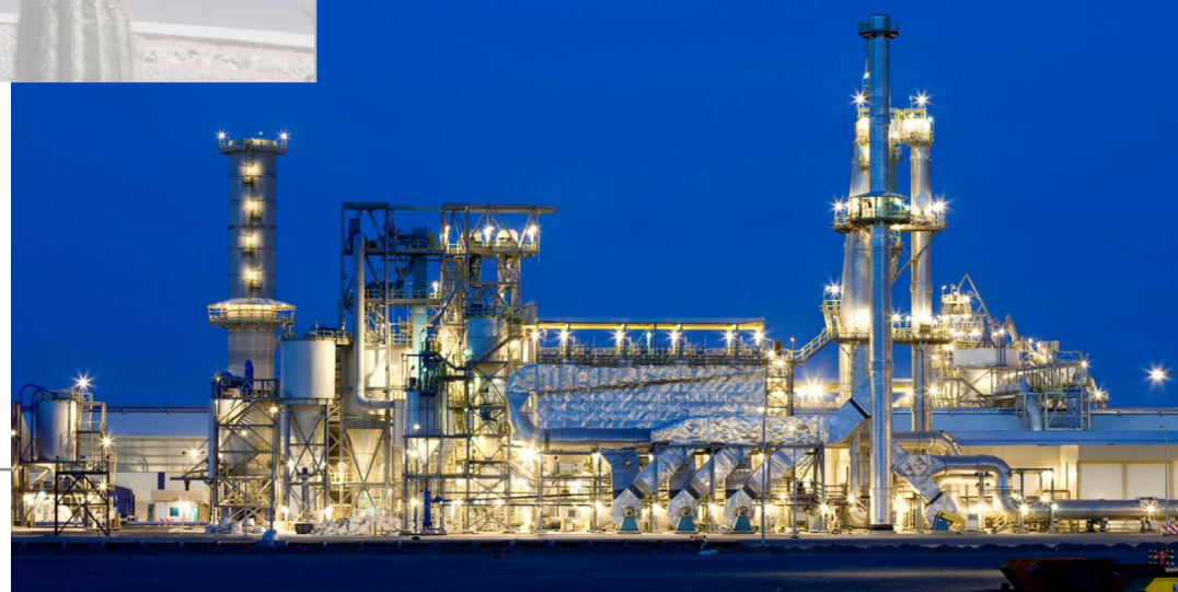
Sohar aluminium plant, Oman (Fives Solios for Rio Tinto Alcan)
